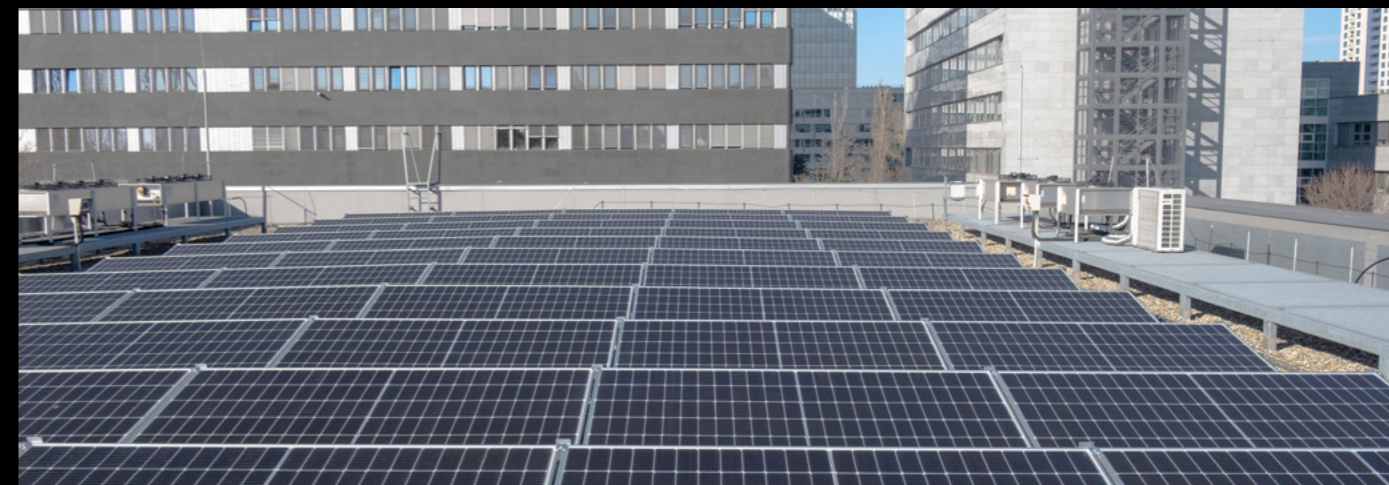
SPP operated photovoltaic power plants at the company's sites in Bratislava and Košice.
